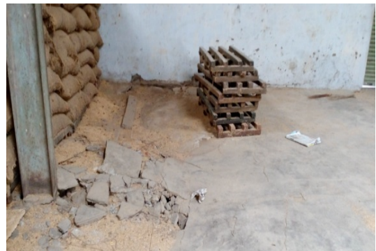
Poor condition of warehouses at Raichur – July 2015
