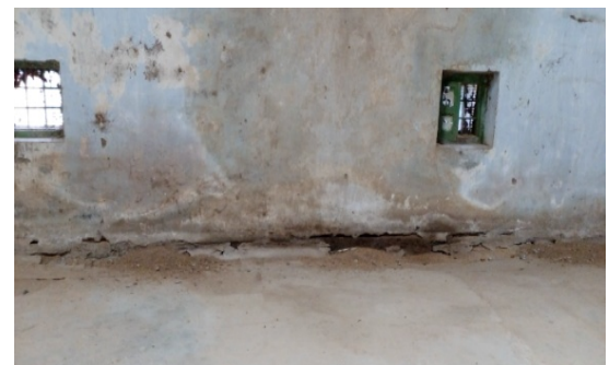
Water seepages and damaged floors at Raichur-July 2015
